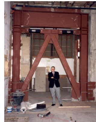
Seismic Dampers installed at the Hotel Woodland, in Woodland, California Force = 100,000 lbs., Stroke = +/- 2 inches Production = 16 pieces
